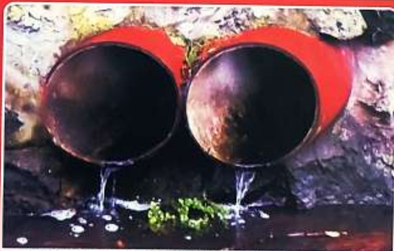
Improper Sewage : Leads to soil contamination
